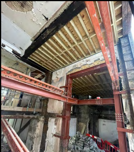
New steel picture frame has been installed in the party wall between 17 and 18 SMS
